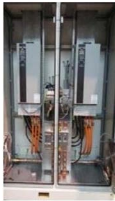
Compressor drives + main power connection
